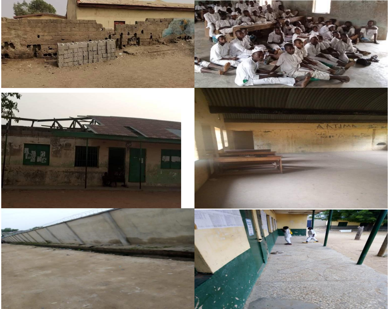
These are some of the school images, which shows the school condition; new classrooms and fence are being built while some classes need to be repaired.
